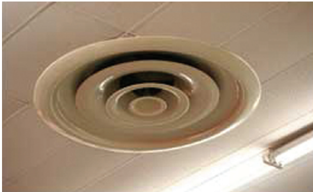
Figure 1. HVAC Ceiling Vent Cover
